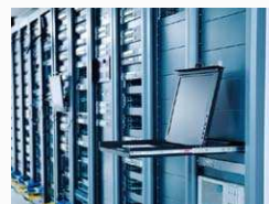
Control Room/ Data Center
